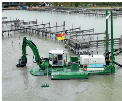
During the first season of maintenance over 60,000 m 3 of soft sediment was dredged out
