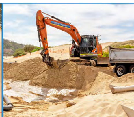
An excavator lifts the sand into trucks to be transported to nearby beaches
