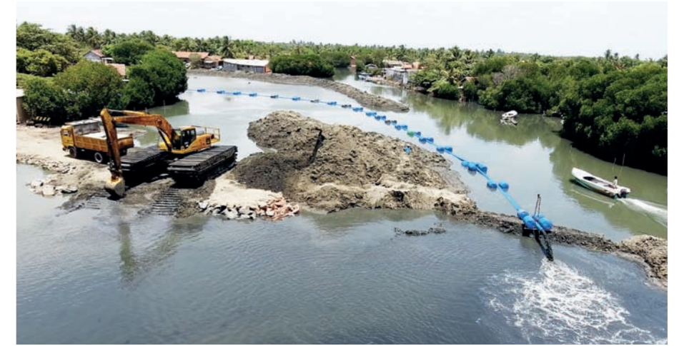
A part of the waterway was separated and used as a settlement pond. Floating excavators helped finalizing the site by lifting the dredged materials onto trucks.
